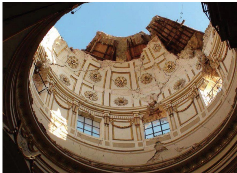
Figure 4. Inner view of the dome after the earthquake of 2009. As can be seen, diagonal cracks separated large portions of masonry which could still stand by virtue of the double curvature of the construction.
