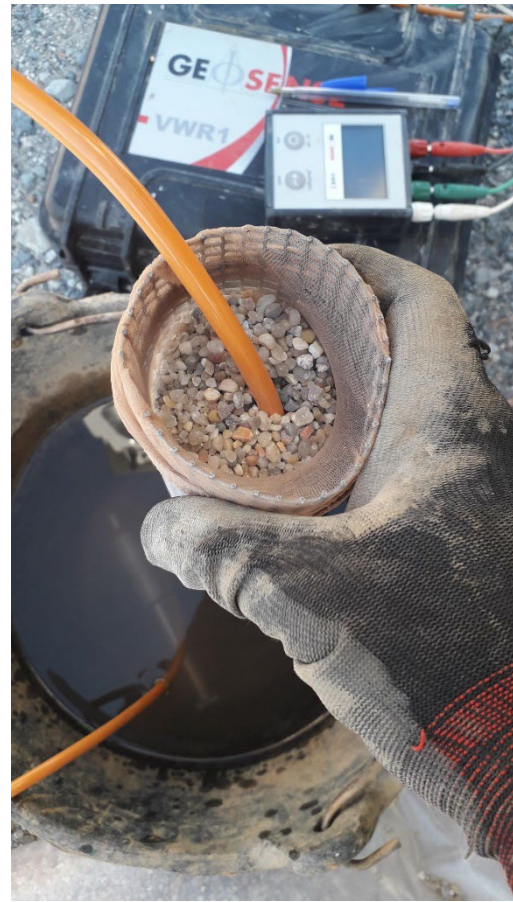
Figure 3. Detail of the granular filter to surround the piezometer following the procedure of the classical approach.
