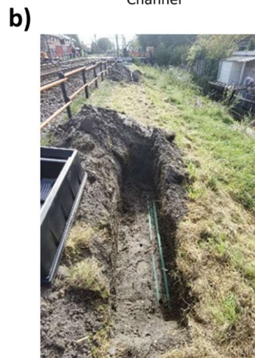
Figure 3. a) Example of a fibre optic recording containing 1 train passage, b) dark fibre cable (green colour cable) buried alongside the Hanzelijn corridor.
