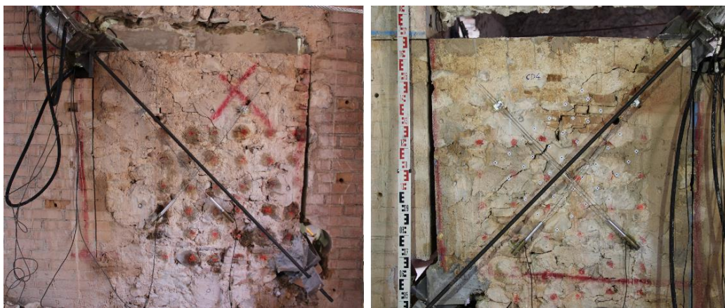
Figure 3: Cracking paths on CD04 specimens after the DC test, side 1 and 2.
