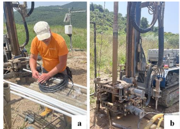
Figure 7. Installation of the CS225 probes on the PVC guide (a) and of the casing (b).
