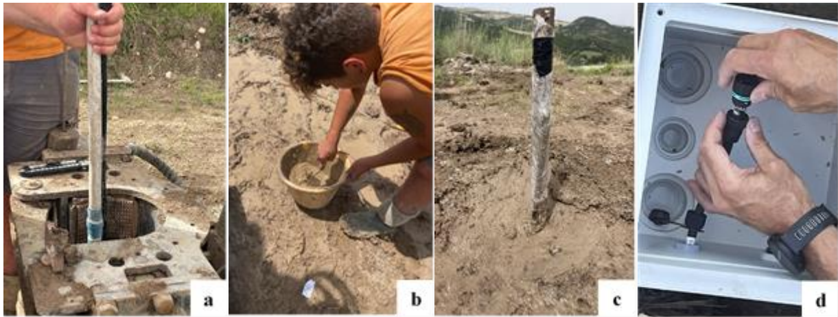
Figure 8. CS225 placement in the borehole (a); filling operation with on-site material (b); the cable ready for the wiring phase (c); wiring procedure (d).
