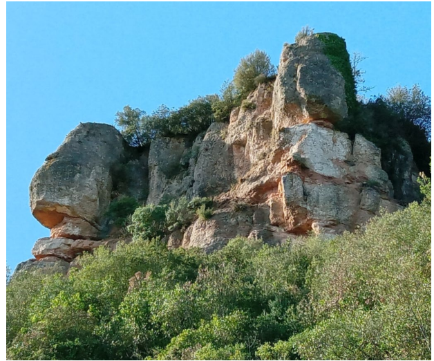
Figure 11. Advanced tests in a block representative of the dynamics of rockfalls in the study area, February 2024. The "Panxo-A" block is the one on the left, hanging vertically over the BP-1103 highway. The TIL90 tiltmeter has been installed at its summit.
