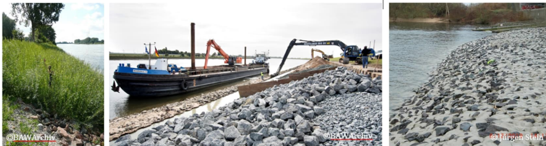
Figure 1: Typical bank protections in inland and coastal areas: technical-biological bank protection (left), loose armor stone revetment (center) and fully-grouted revetment (right)
