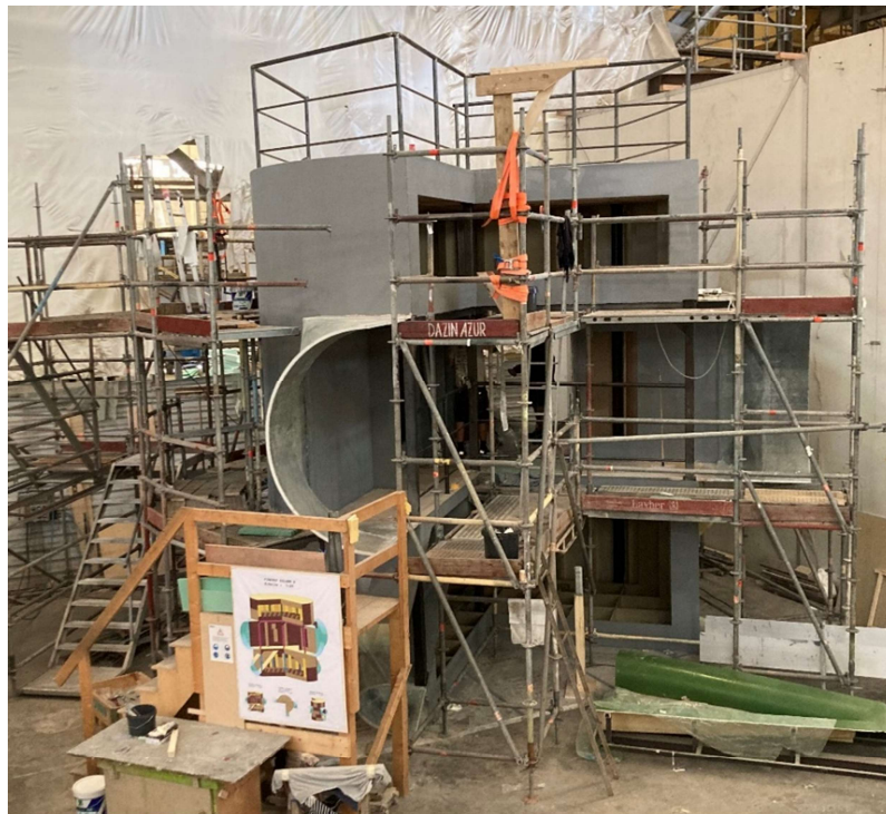
Figure 18 : Column without finishing
