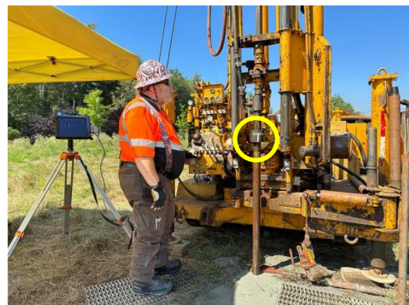
Figure 1. MWD equipment operated by a driller in Newington, NH. The yellow circle highlights the wireless torque sensor installed directly at the top of the drill string.
