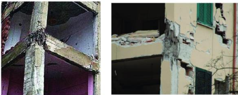
Figure 2: Cracking of structural joints after an earthquake (Moslam, 2013)
