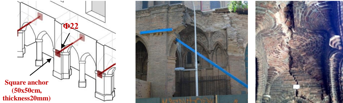
Figure 1: External gallery walls of Basilica del Salvador: (a) Tie-rods device to prevent the OOP mechanism, (b) collapse of external gallery pillars, and (c) deep crack in the arches and vaults.
