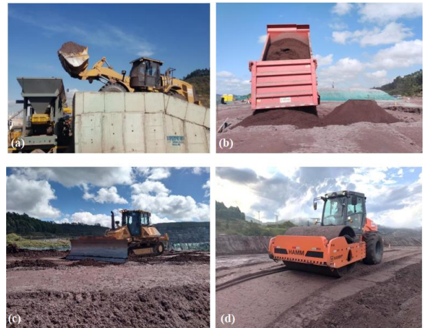
Figure 1. Construction of the experimental piles: (a) tailings collection, (b) deposition of the tailings, (c) spread of the tailings, and (d) compaction.
