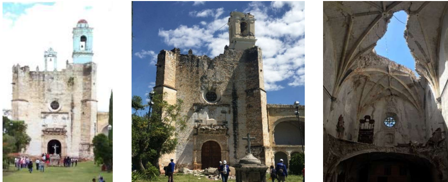
Figure 4: Left: Before the earthquake, May 2017 [13]. Center: After the earthquake, Oct 2017. Right: Damage sustained by the ribbed vault caused by the collapse of the top part of the bell tower, Oct 2017.
