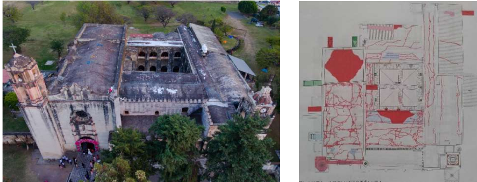
Figure 1: Left, before earthquake, Dec 2016 [12]. Right, after earthquake, roof plan showing damages. Red denotes severe damage and fractures. Pink shows missing bell tower. Blue denotes partial collapse of vaults and in green is the detachment and presence of microflora. May 2019 [5].
