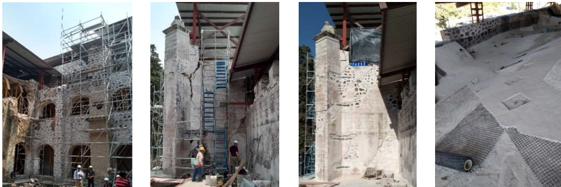
Figure 3: Left: Reconstruction and consolidation of walls and buttresses in the courtyard, Dec 2019. Two central images: Bell tower with damages, May 2019, and after repair by integrating horizontal large volcanic stones, Dec 2019. Right: Rehabilitation of the roof vault by adding carbon fibres in a cross pattern, Dec 2019.
