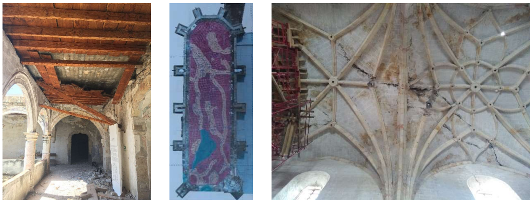
Figure 5: Left: Damage caused by reinforced concrete roof in the cloister, Oct. 2017. Central: Proposed intervention to the nave. Blue indicates reconstruction with similar material. Yellow indicates consolidation at the crack locations. Red only requires a waterproof coating using traditional methods. [14] Right: Main fractures to ribbed vault, May 2019.
