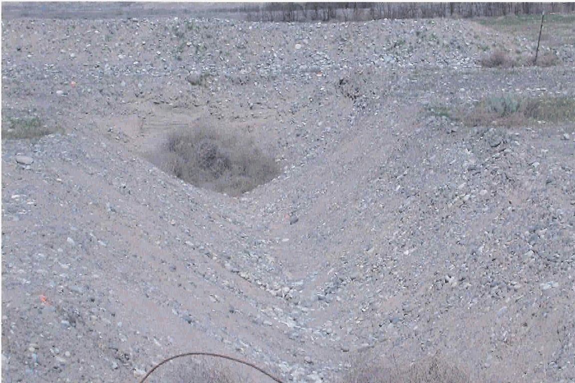
100-F-26:10 Waste Site Excavation (smaller excavation to the north; looking north; April 18, 2007).
