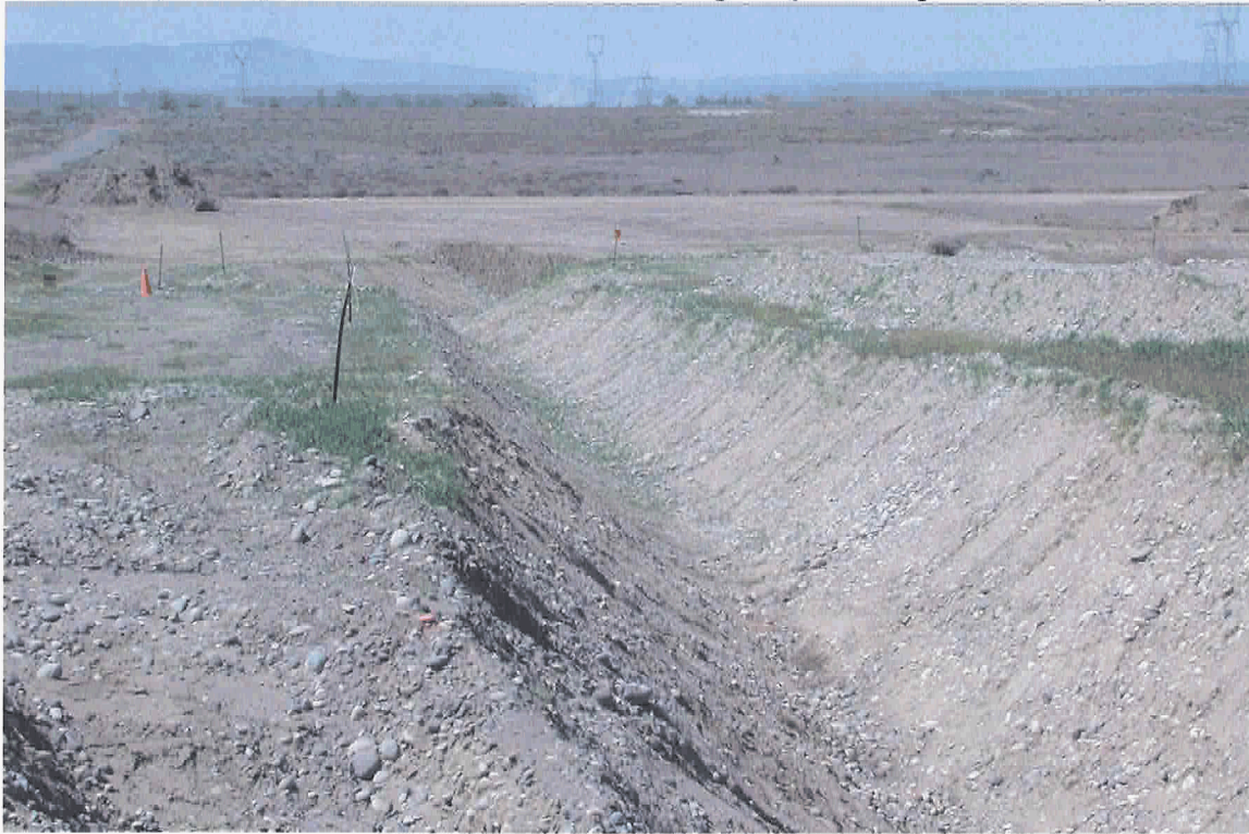
100-F-26:10 Waste Site Excavation (looking west toward former 1607-F3 septic system; April 18, 2007).
