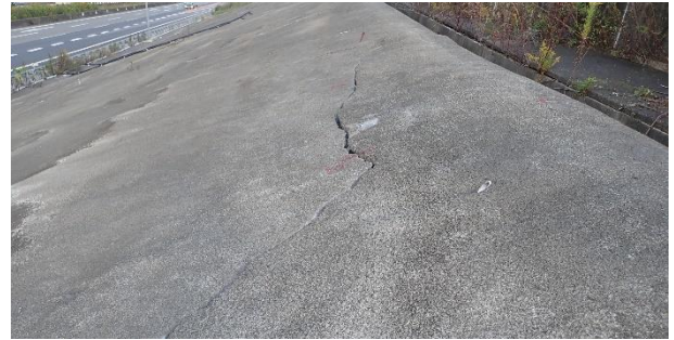
Figure 10. Cracks of the mortar sprayed slope at the lower part of the slope due to squeezing deformation.
