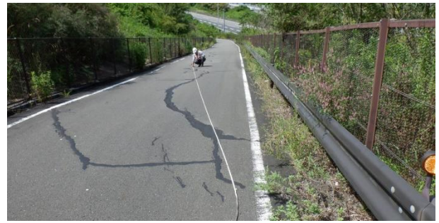
Figure 9. Joint cracks on the side road.
