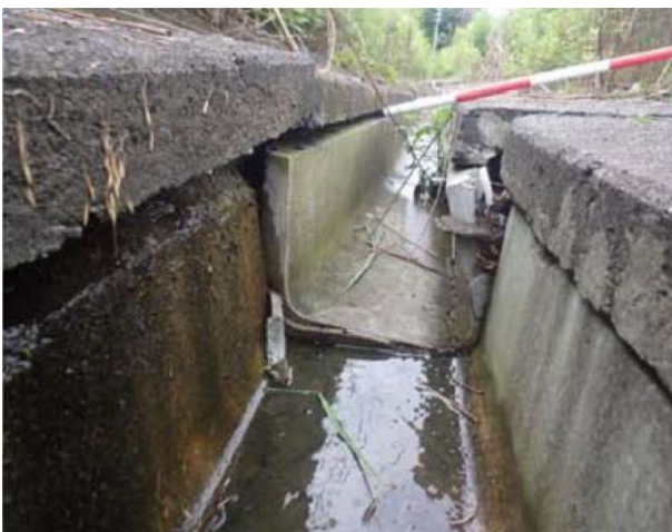
Figure 8. A waterway block subjected to squeezing at the lower part of the slope.
