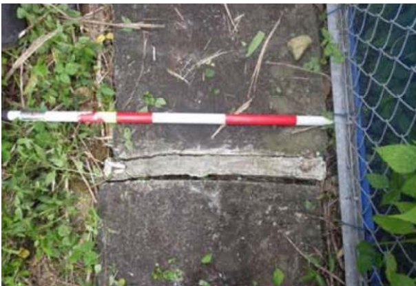
Figure 7. A vertical crack along the mortar joint of the waterway at the upper part of the slope.
