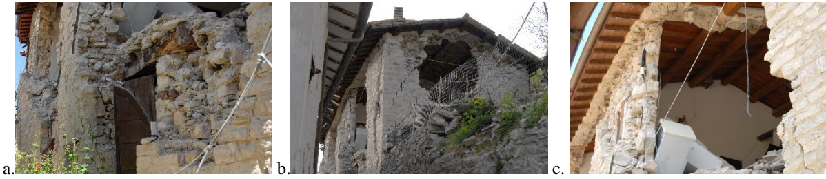
Figure 3: Examples of poor seismic behaviour in a strengthened masonry building, CSN: a) Not effective tie rods on bad quality masonry; b) overturning of last storey and c) of internal bearing walls due to r.c. curbs and to excess of stiffness and weight of reinforced timber roof
