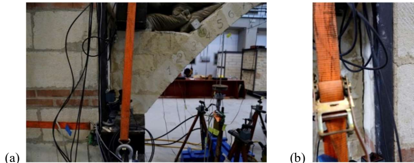
Figure 9: The crack hinges: (a) Front view and (b) back view of the masonry vault
