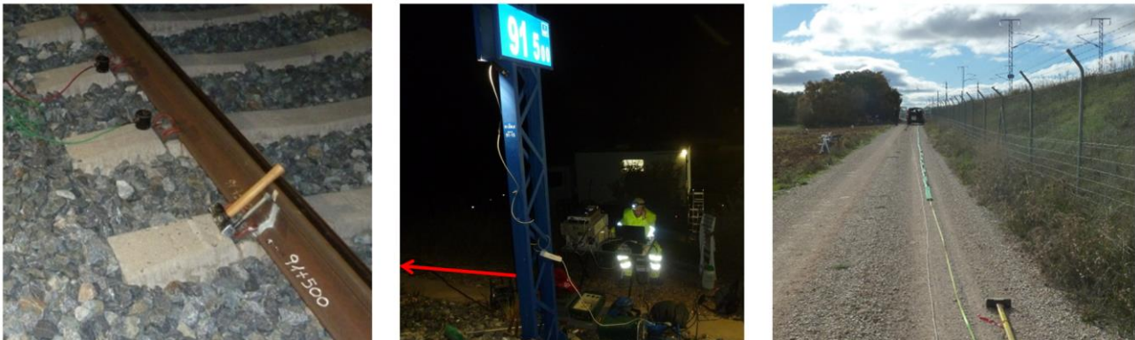
Figure 5. Photos taken during the performance of the tests carried out to study the ballast (left); the embankment (center) and the natural ground.
