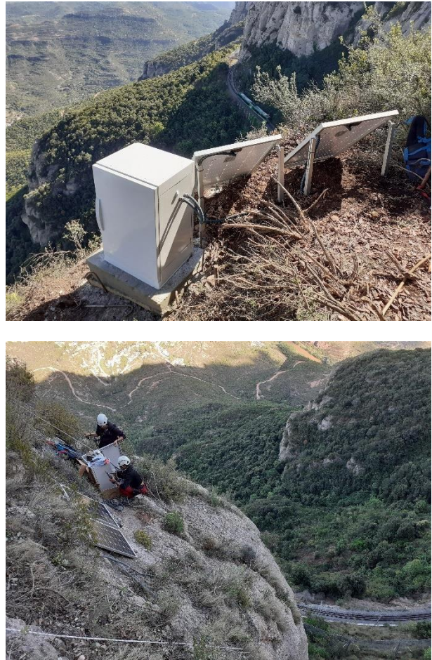
Figure 2. Installation on site of the monitoring devices on the massif (upper) and the block (lower).
