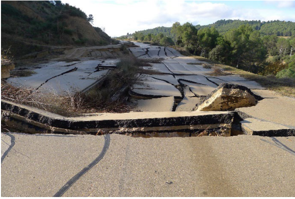
Figure 2. Failure in “zone 5”.
