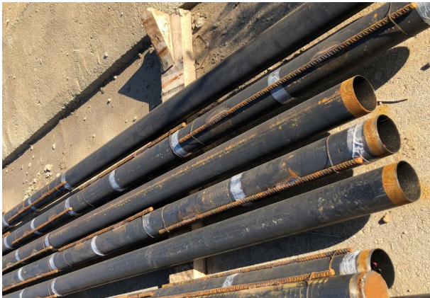
Figure 20. Corrugated bars welded to the protective tubes of the grouted bulb of anchors
