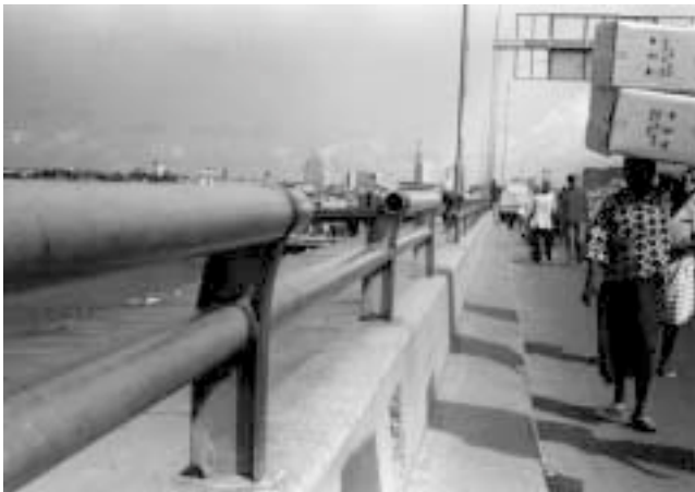
Photo 3 Broken bridge railings/barrier. Pedestrian are forced to walk along the road with moving vehicles
