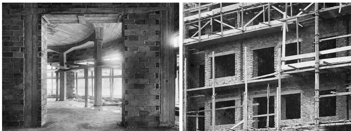
Figure 6: Novocomum under construction: one can see the outside and internal walls in perforated brick (ATCo).
