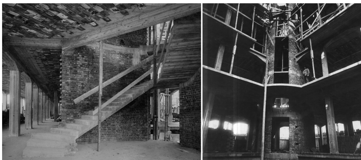
Figure 7: Novocomum. Worksite photographs showing the stairwells with walls of solid brick (ATCo).
