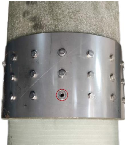
Figure 127 – Post-testing inspection from the outside (specimen #2)
