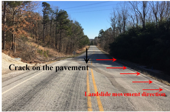
Figure 2. A sample longitudinal crack observed on the pavement.
