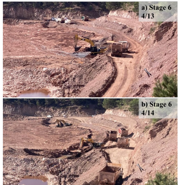
Figure 11. a) Excavation of fluid-like tailings during stage 6, b) Excavation of soil-like tailings during stage 6.
