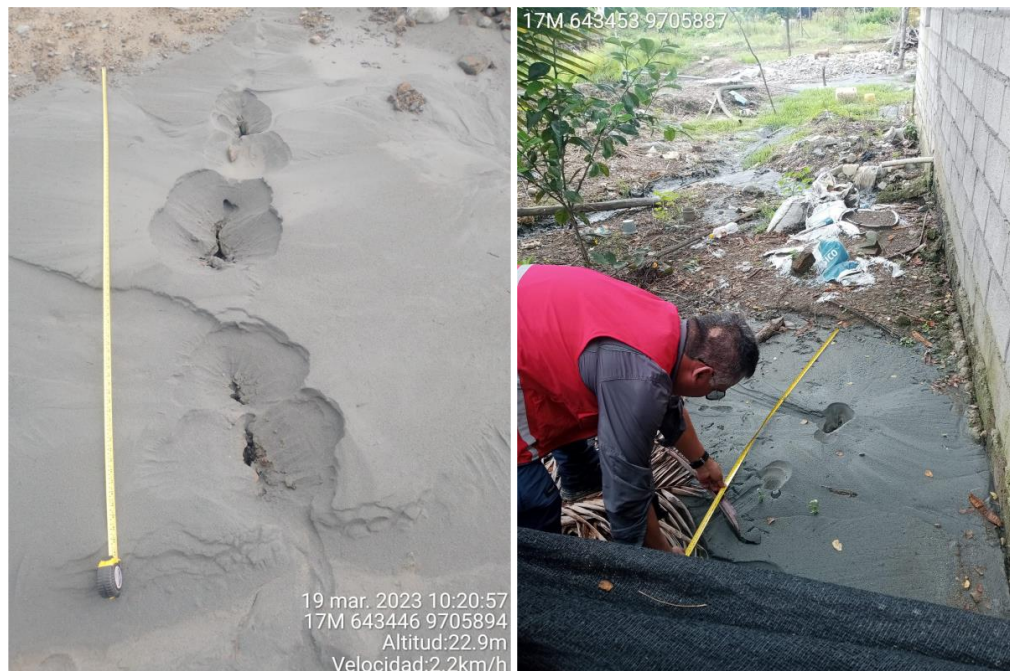
Figure 1. Ground Cracking, sand boils and ejected soil as a liquefaction evidence in Puerto Baquerizo.
