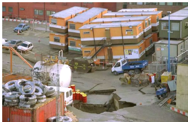
Figure 1. Tunnel roof collapse in Heathrow central area during the construction of the rail link to Paddington (See Airnews copy)
