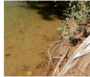
Figure 3. Riverbank erosion at the abutment
