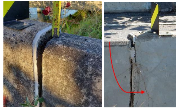
Figure 7. 2019 Concrete barrier movement abutment of the heritage bridge
