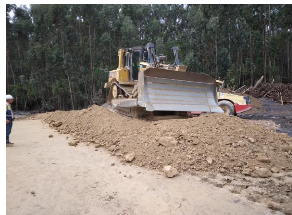
Figure 5. Brown schists in the earthfill.
