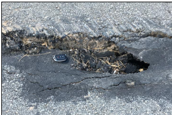
Figure 2. Displacements observed on the external asphalt pavement.
