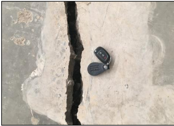
Figure 1. Crack observed on the inside concrete floor.
