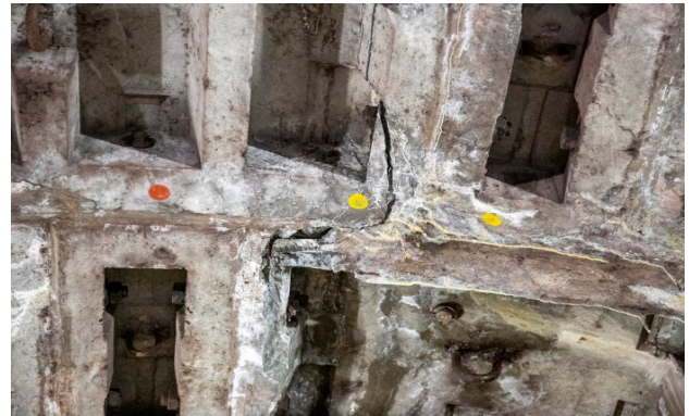
Figure 9. Cracks in the emergency section of the metro ( https://telegraf.com.ua/kyiv/2023-12-08/5821615-pidtoplennya-i-zakrityta-metro-u-kyievi-shcho-vidbuvaetsya-naspravdi-i-skilki-trivatime-transportniy-kolaps )
