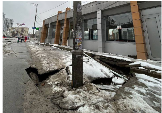
Figure 10. Cracked asphalt and dips above the emergency tunnel ( https://telegraf.com.ua/kyiv/2023-12-17/5822993-nad-zatoplenoyu-stantsieyu-metro-u-kyievi-nova-np-eksklyuzivni-foto-ta-video )
