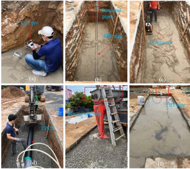
Figure 3. (a-c) TRT set up for natural sand: (a) measurement of thermal properties of soils using KD2 Pro, (b) steel pipe GHE backfilled with sand, (c) compaction of sand, (d-e) TRT set up for prepacked concrete: (d) installing UPCS, (e) The trench filled with gravel, (f) The trench filled with grout
