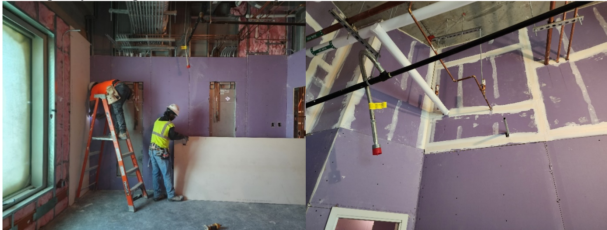
(a) A two-man crew measuring, cutting, and installing drywall boards on a construction site
